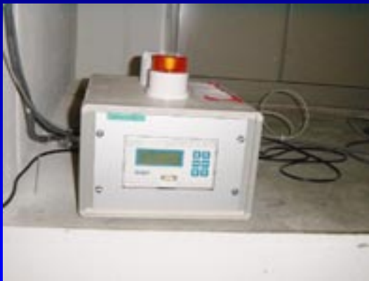
Gas Alarm units
